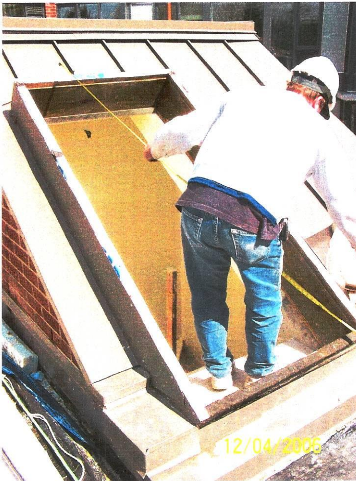
#4- Installer is in the process of measuring a rough opening for squareness.
