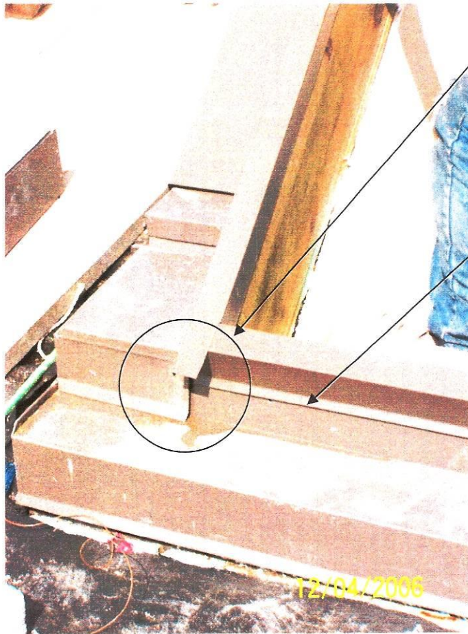
#7- Close-up view of excess jamb flashing at sill area for overlap of sill flashing. Note – view also shows sill flashing kick-out detail to deflect rain water from the curb area.
