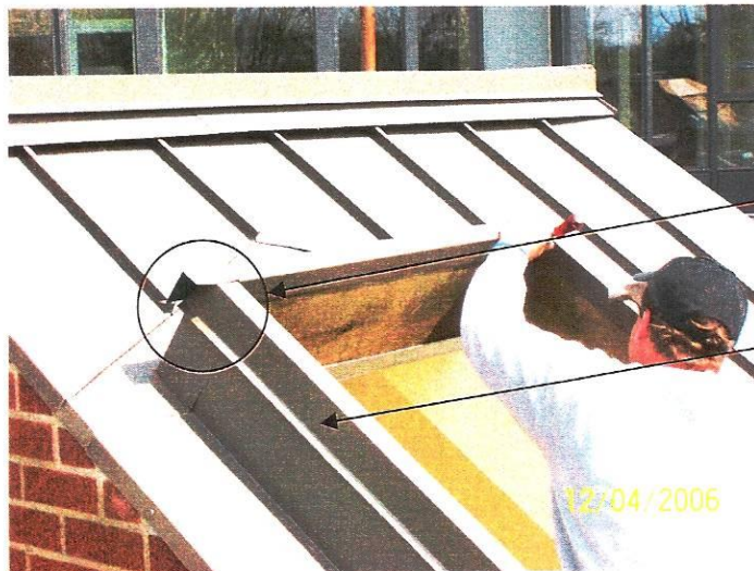
#8- Installation of head flashing. Installer has notched the head flashing and is punching a hole in the end for the fastener.. Note – the excess flashing on the end will be cut and folded to create a ‘shingle’ water deflection seal. Also note the jamb flashing ‘kick-out’ detail for deflection of rain water away form the curb.
